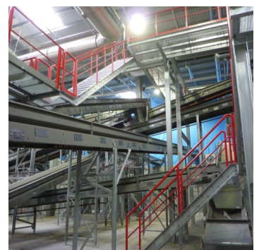
Waste separation equipment
