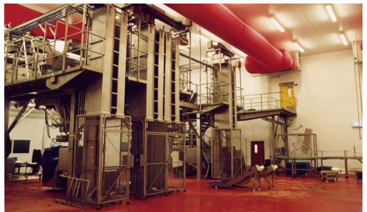
High care bagging area
